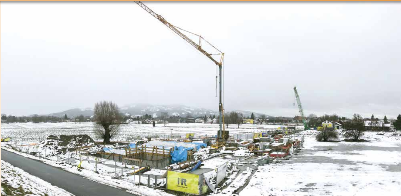
Das Pumpwerk in Fussach
